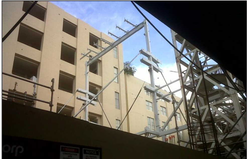
The framework of the front of the building where the cross will be illuminated.
